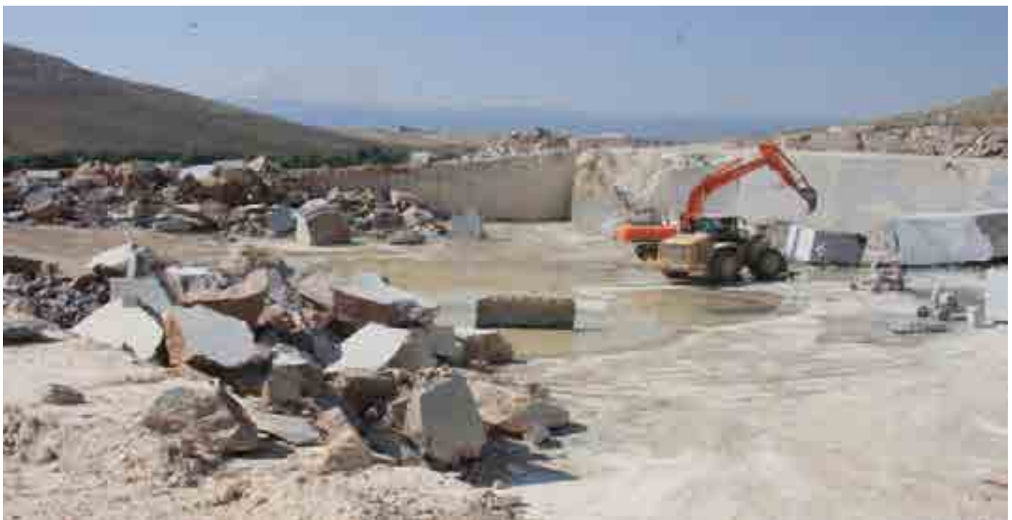
A photograph of a cement construction area with large pieces of debris spread out throughout the landscape. Bulldozer on the right, In use. BESMAR Marble Quarry near Karaköy village, Konya, Turkey.
